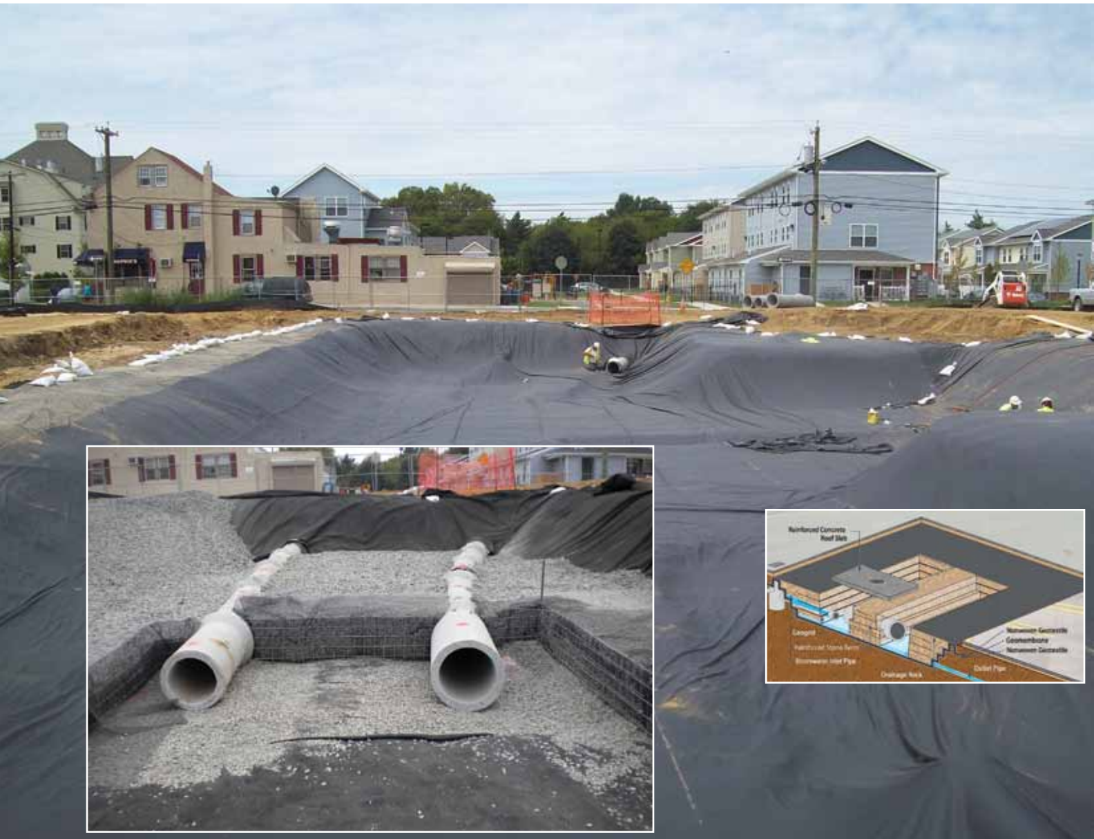
PVC geomembrane installation over underground chamber. Inset: Perimeter wall construction at pipe penetration. Schematic of patented geosynthetic based underground stormwater detention system.
