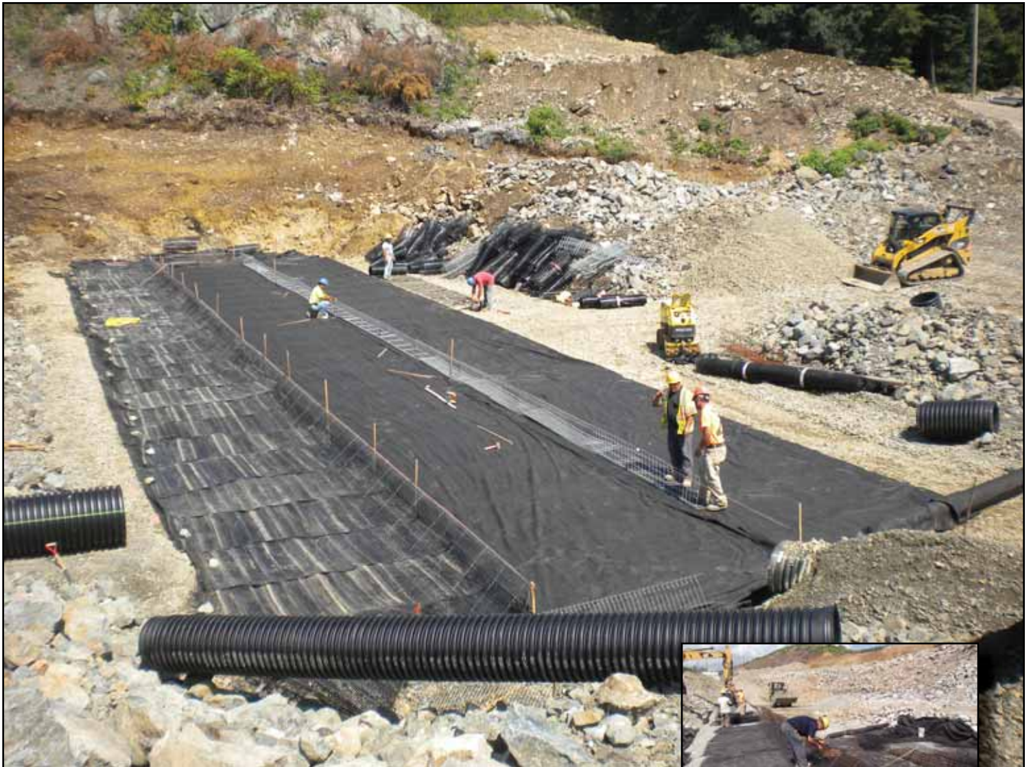
Above: Site preparation: chamber wall alignment and construction atop the geotextile liner. Inset: chamber wall construction: Support struts stiffen the welded wire face form with wrap geogrid draped over top and the reinforcement geogrid embedded into the stone backfill.
